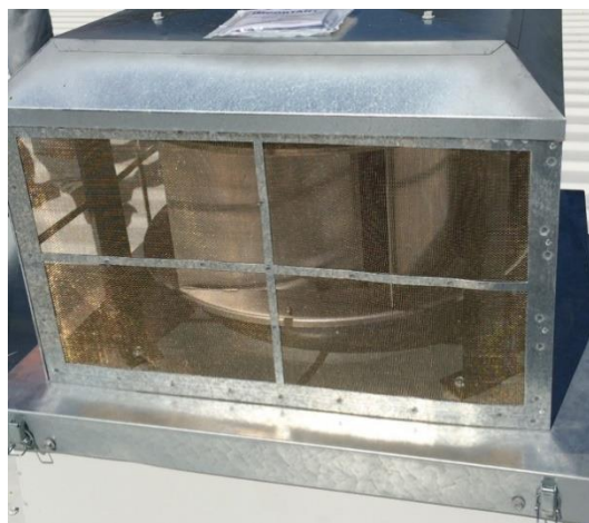
Figure 11 – Ember guard roof exhaust system
