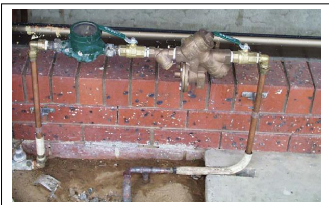
FIGURE 3 - REDUCED PRESSURE ZONE DEVICE - RETROFITED FOR CONTAINMENT PROTECTION
