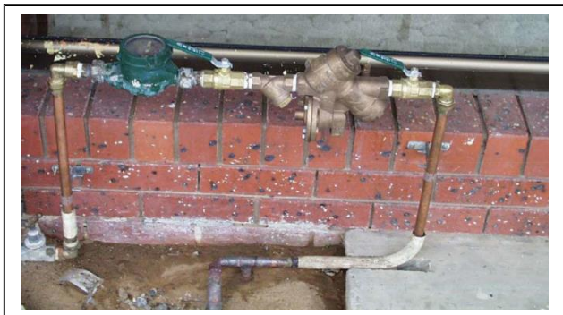
FIGURE 3- REDUCED PRESSURE ZONE DEVICE- RETROFIT FOR CONTAINMENT PROTECTION
