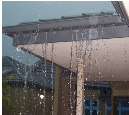
An example of rainwater overflowing from the eaves gutters during a storm event.
