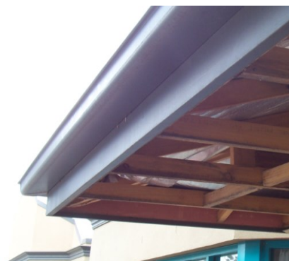
An example of a roof requiring new eaves linings after damage caused by water overflowing from the eaves gutters.
