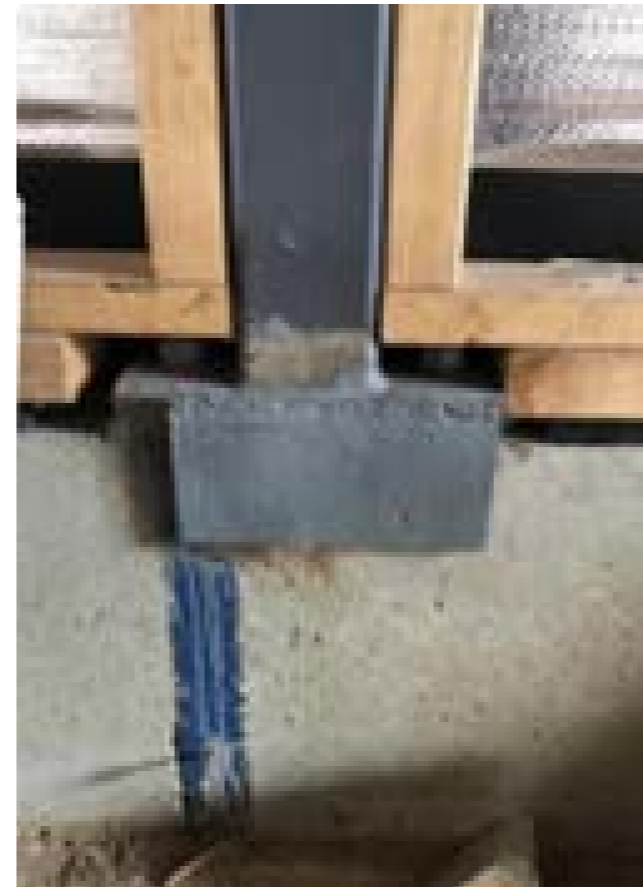
P2 posts were not installed as per the engineering documents and bolted connection from above fell within square hollow section.
