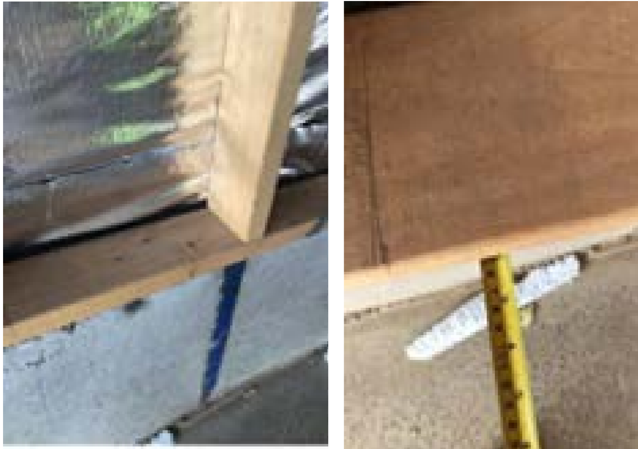
Timber bottom plates overhanging slab by 50mm.
