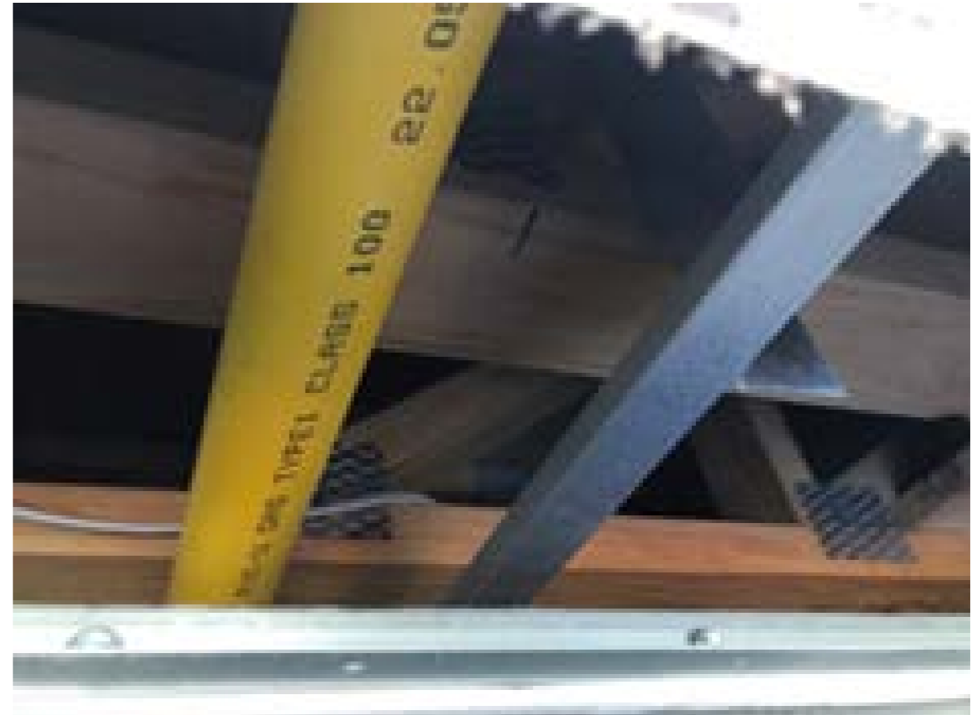
Non-compliant plastic gas pipework material used below a building.
