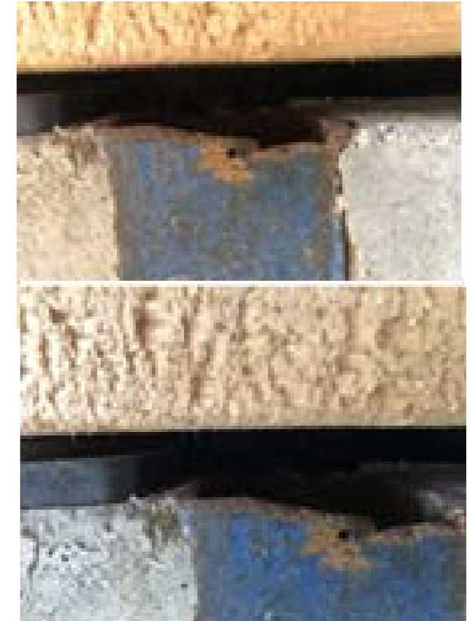
Bottom plates installed on large amounts of packers with inadequate fixings.
