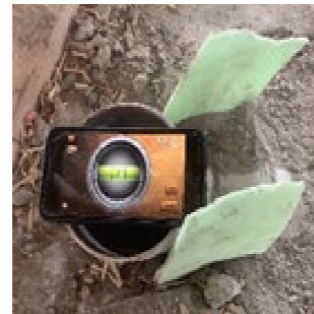
Gradient of drain going backwards contrary to AS 3500.2:2021.clause 3.4.1
