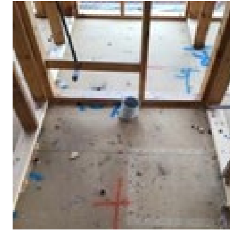
Some risers are not installed parallel, pipe work shall be in the same alignment and grade as the preceding pipes or fittings. AS/NZS 2032:2006 Clause 4.2.3
