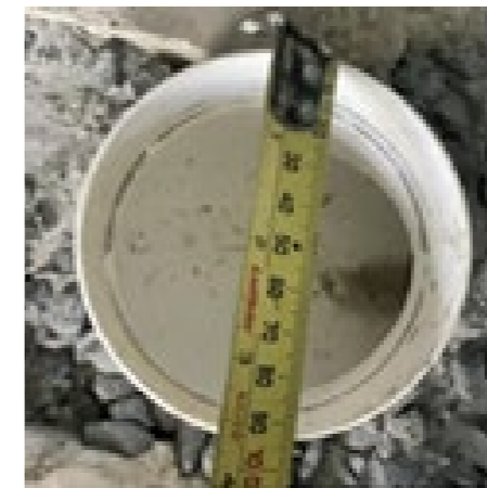
90mm PVC piping. not suitable for sanitary drainage systems contrary to AS/NZS 3500.2:2018 clause 2.3 and manufactures installation specifications.
