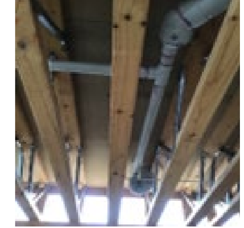
Incorrect junctions and venting of the sanitary drains contract to AS/NZS 3500.2:2021 clause 9.5.2 & 9.2.2 AS/NZS 3500.2:2021 Clause 6.6.2.3
