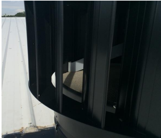
Figure 4 – Ember guard in vent
