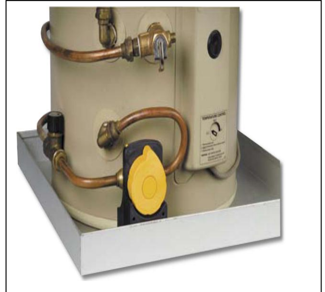
FIGURE 2 - EXAMPLE OF A COLD WATER SHUT OFF DEVICE IN AN UNDRAINED SAFE TRAY
