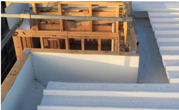
Image 1 - Box gutter installed with a change in direction is NOT PERMITTED .
